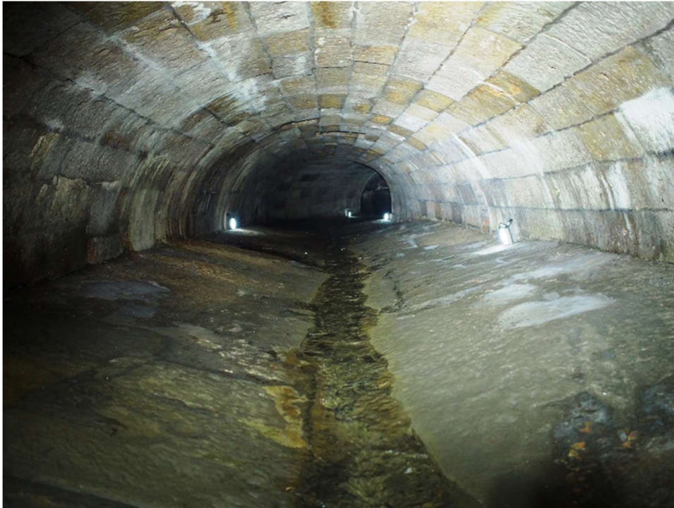
Figure 6-32 – The sandstone masonry arch section of the Tank Stream. Source: Sydney Water
